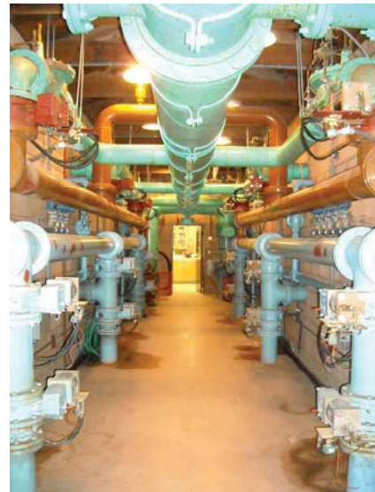
City of Yreka water treatment plant, photo taken 5/12/2009
